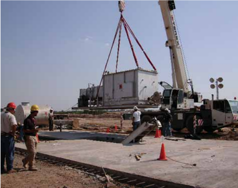
A trash-burning incinerator is installed at Forward Operating Base Warhorse, Iraq, through a LOGCAP contract.
